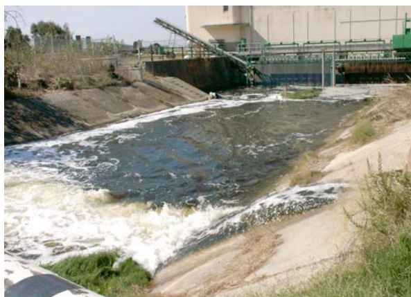
Figure 3: Canale delle acque basse and pumping station
